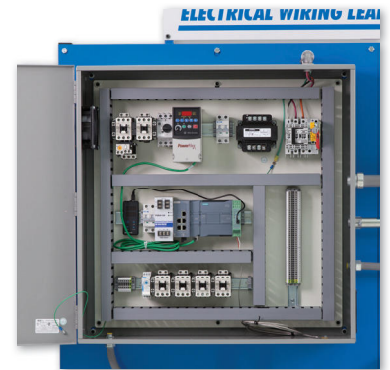
VFD & PLC Mounted in Panel
