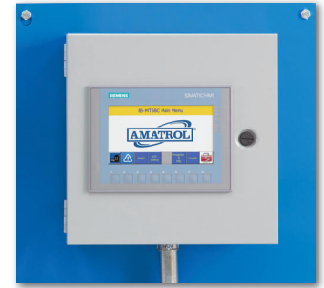
Siemens HMI Panel Installed on the Electrical Wiring System
